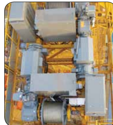
HOISTING & LUFFING GEAR
